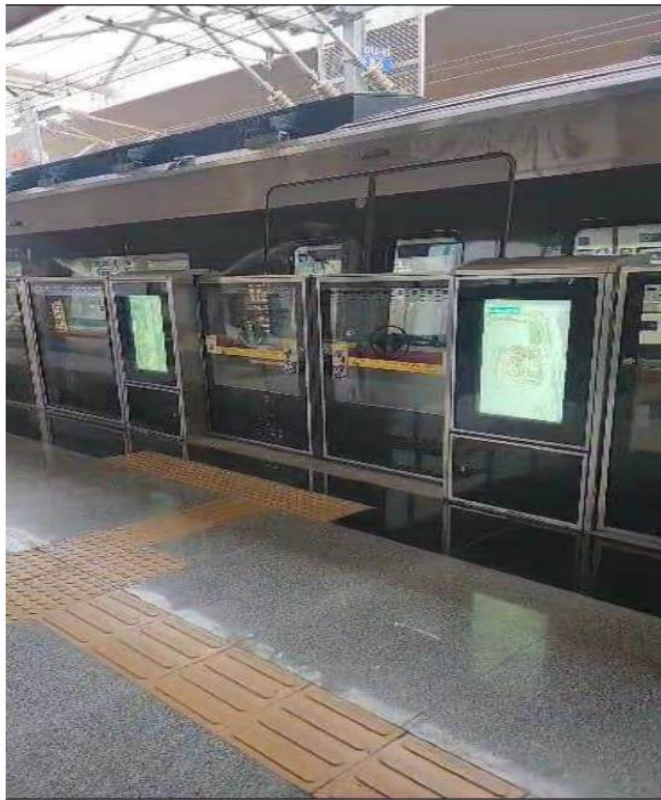
Platform Screen Doors
