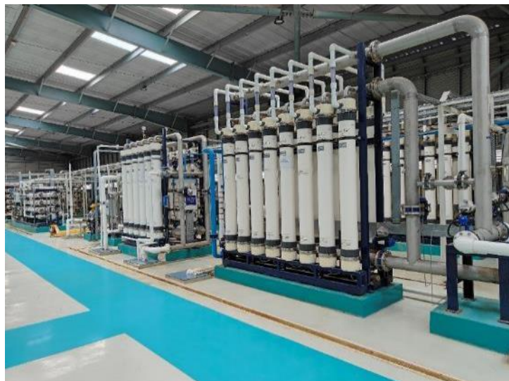
Ultra-pure water generation plant at Unit II
