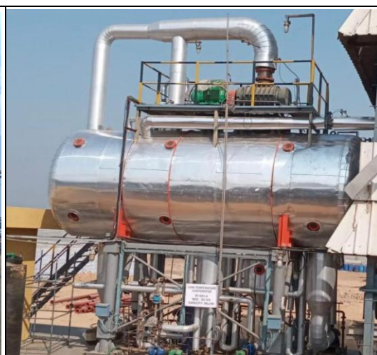
MVR_waste water treatment facility
