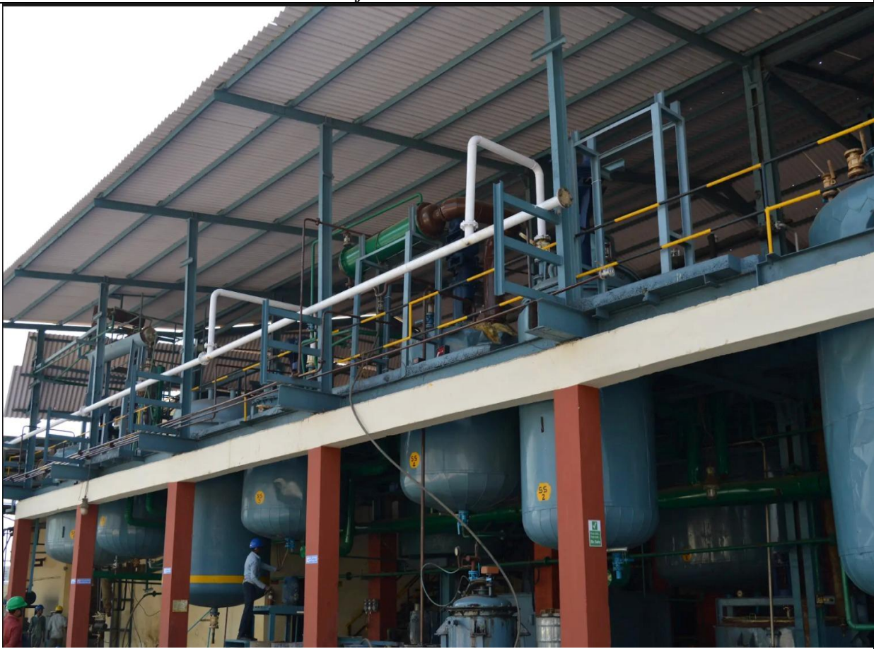
Reactors in Plant 3
