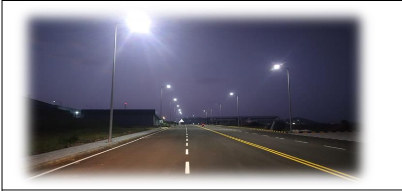
External Lighting - Indospace - Chakan - Pune
