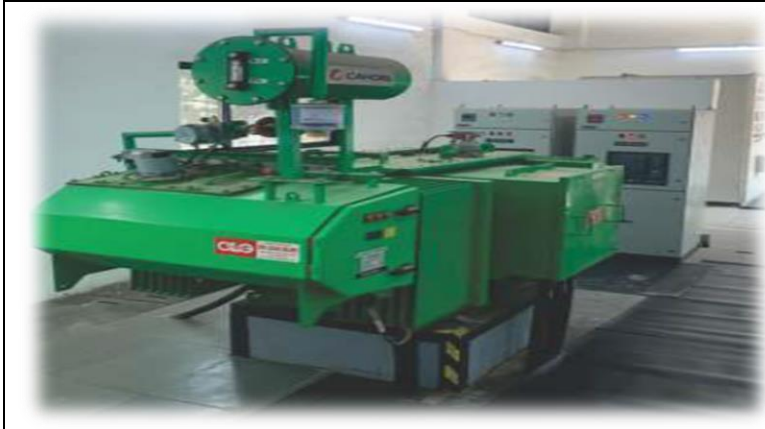
HT Sub Station Works - M/s. Mastek Ltd - Mahape - Navi Mumbai
