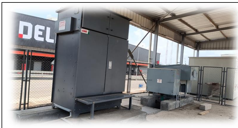
HT Sub Station Works - Welspun One Logistics Parks Pvt. Ltd. - Bhiwnadi
