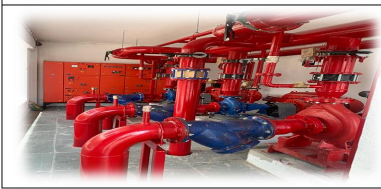
Fire Fighting System - M/s. Mastek Ltd - Mahape - Navi Mumbai
