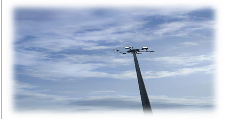
High Mast Poles - Indospace - Chakan - Pune
