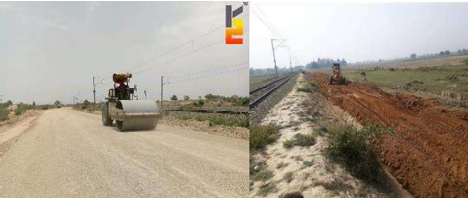
Vindhya Telelinks Limited Power Distribution Varanasi FY 2017-18
