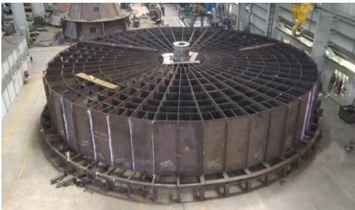
TYPE OF JOB - Air Pre Heater Industry – Power Plant HEIGHT And WIDTH – 2.8 Meter and 16 Meter WEIGHT – 140 MT approx. in assembled condition
