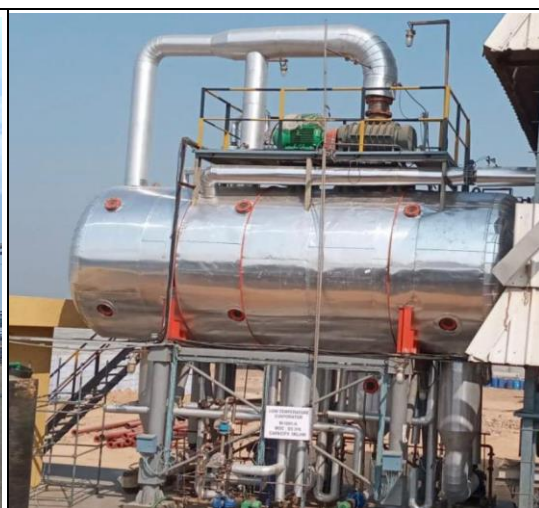
MVR_waste water treatment facility
