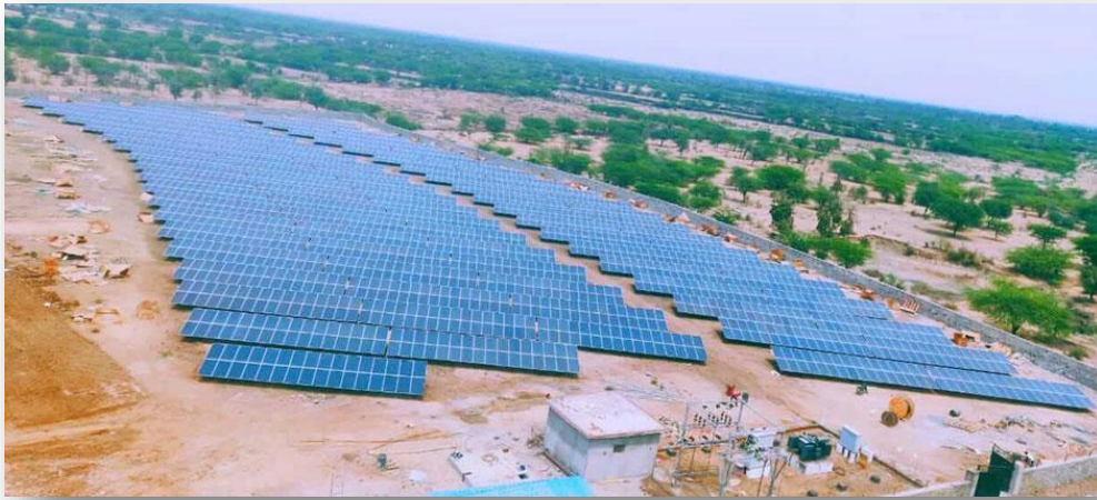
933 kW Captive Solar Plant at Bhilwara, Rajasthan
