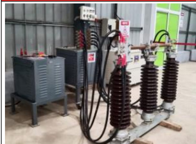
HV DISCONNECTOR STRUCTURE
