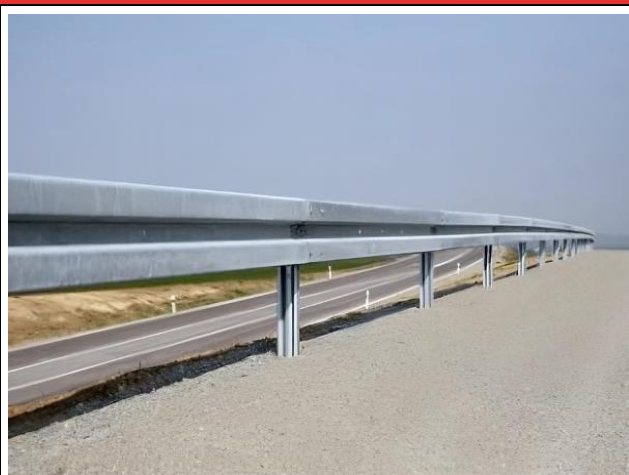
METAL BEAM CRASH BARRIER
