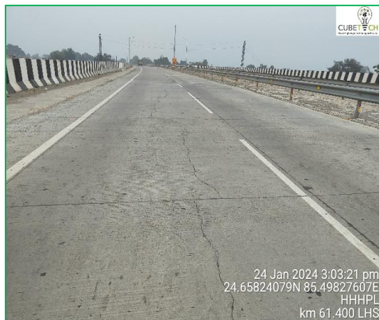
Figure: Longitudinal Cracks
