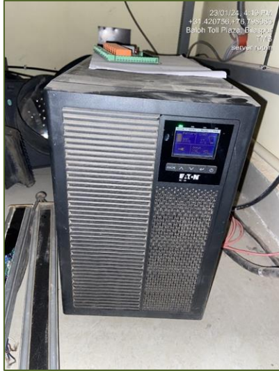
Figure 3-21: UPS at Server Room.
