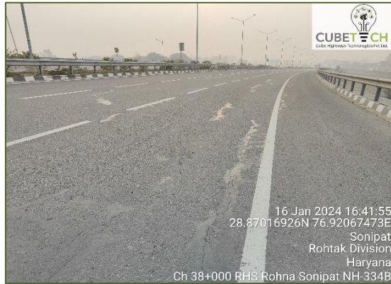
Figure: Longitudinal Cracks
