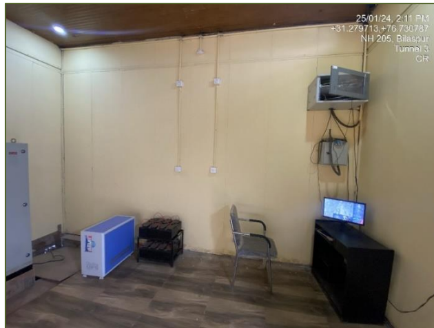
Figure 3-49: Tunnel-3 Control Room.
