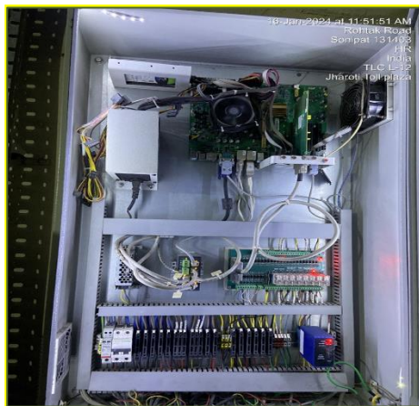
Figure 3-9: Toll Lane Controller at Tunnel
