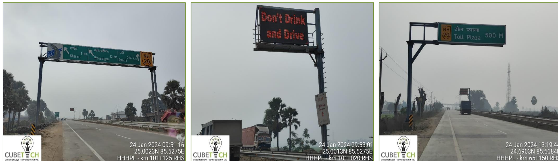
Figure 3-6: Overhead & Cantilever Gantry boards and VMS
