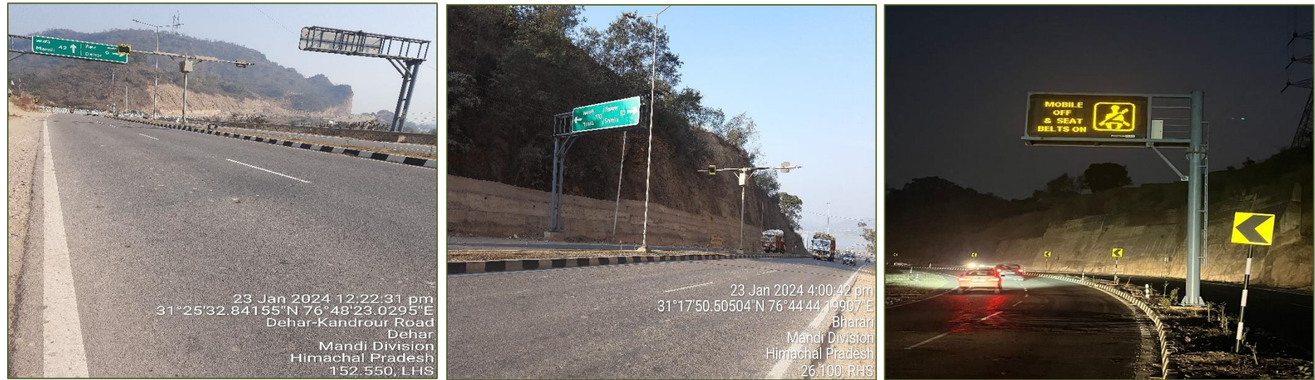
Figure 3-5: Overhead & Cantilever Gantry boards and VMS
