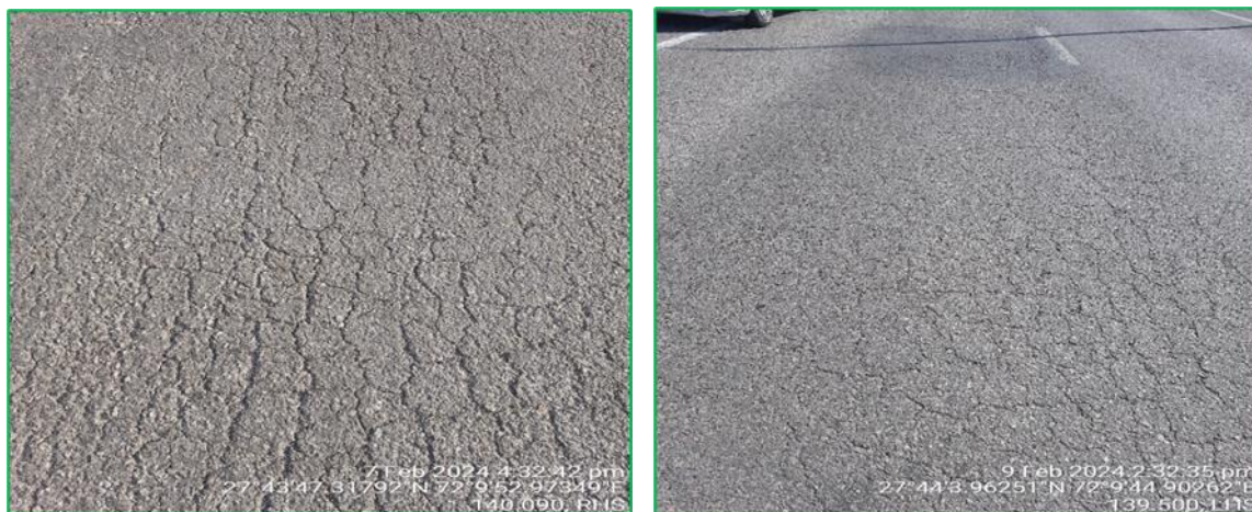
Figure: Alligator Cracks
