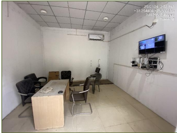
Figure 3-47: Tunnel-2 Control Room.
