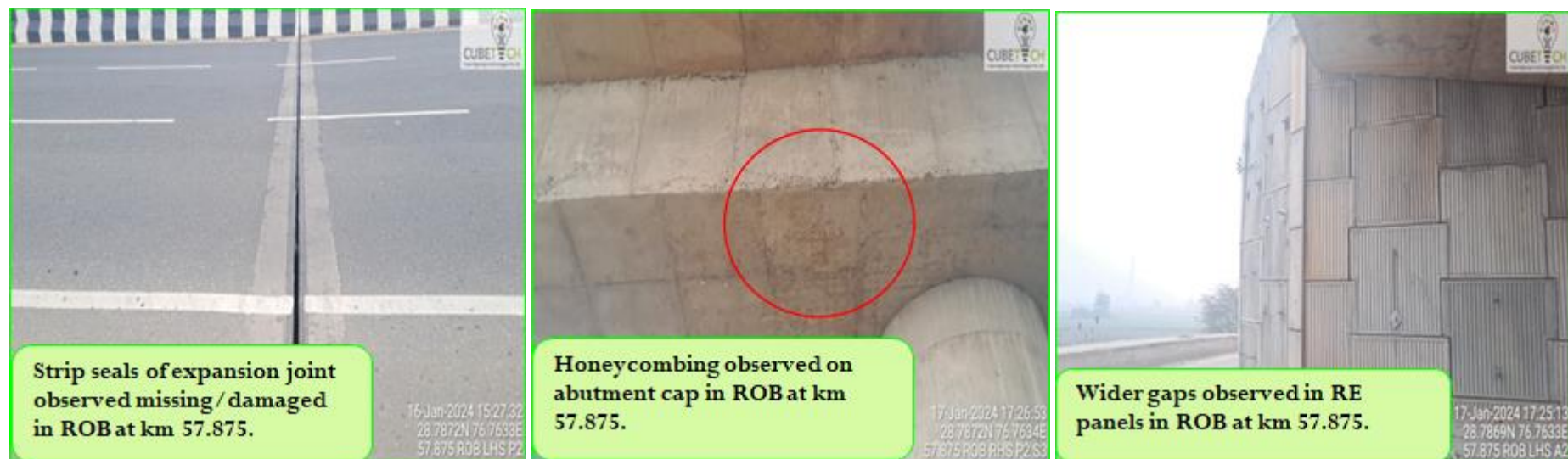
Figure 4-2: Condition of ROB
