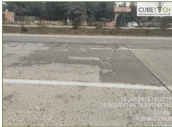
Figure: Tranverse Cracks
