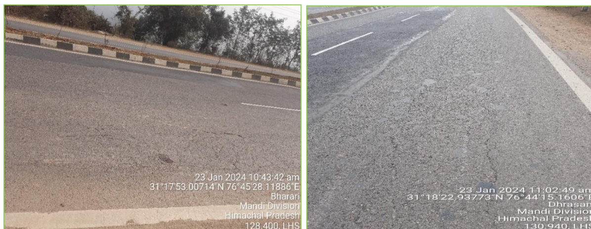
Figure: Alligator Cracks
