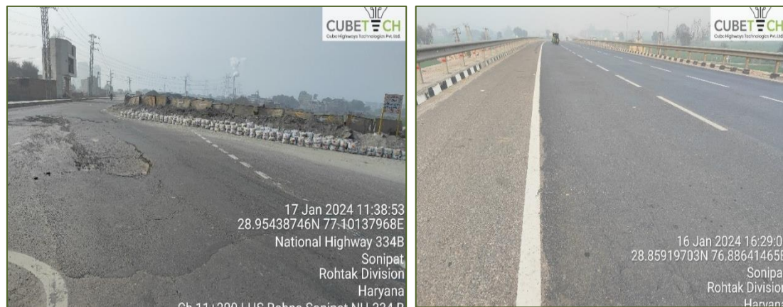
Figure: Alligator Cracks
