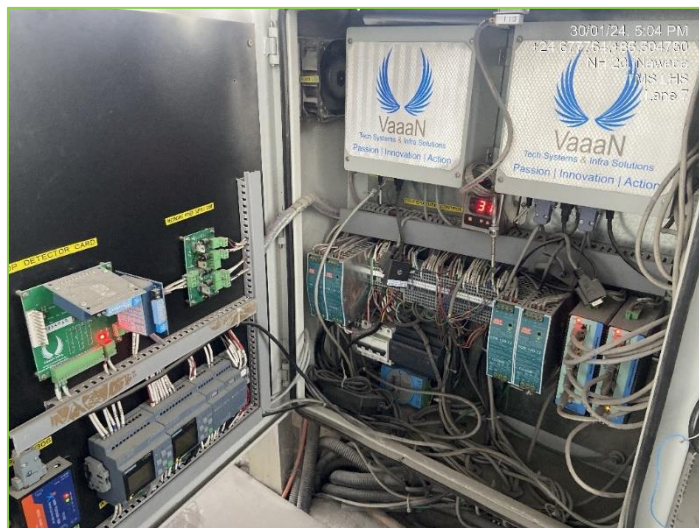
Figure 3-16: Toll Lane Controller inside Booth
