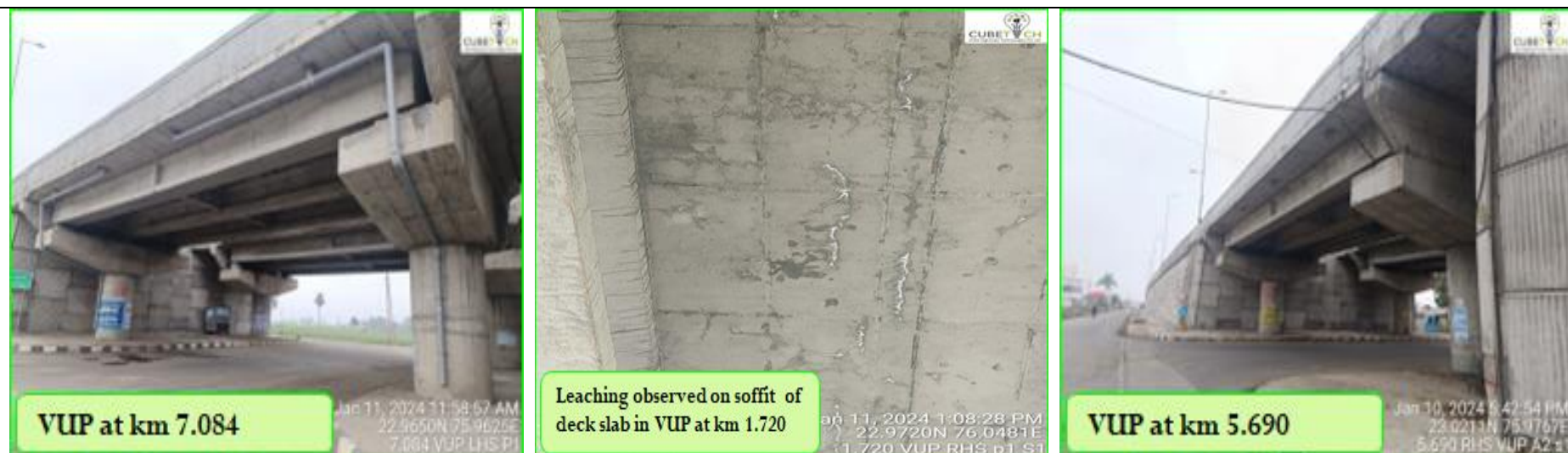
Figure 4-5: Condition of VUPs
