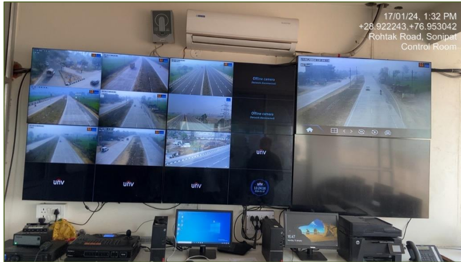
Figure 3-30: ATMS Control Room Equipment.
