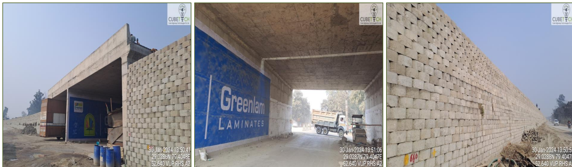
Figure 4-5: Condition of Vehicular Underpass
