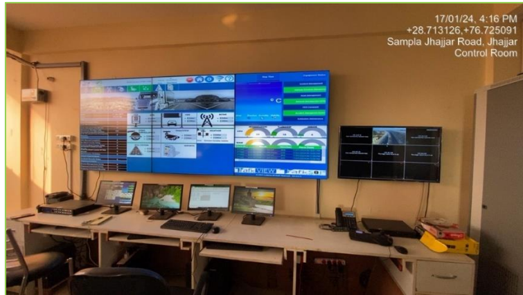
Figure 3-31: ATMS Control Room.
