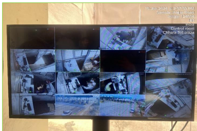
Figure 3-20: CCTV screen at the Toll Plaza Control Room.
