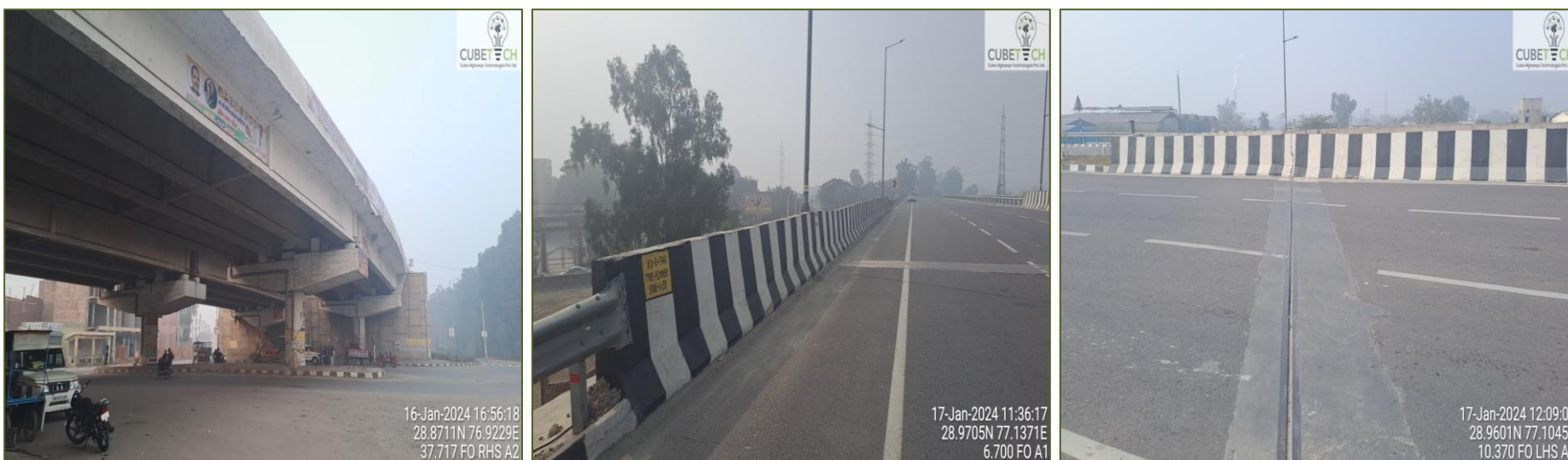
Figure 4-3: Condition of Flyover
