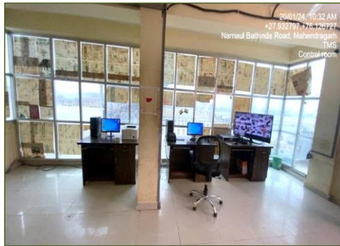
Figure 3-18: Workstations at Control room.
