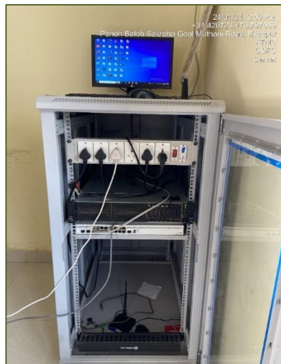
Figure 3-39: ODFS Server with Rack.
