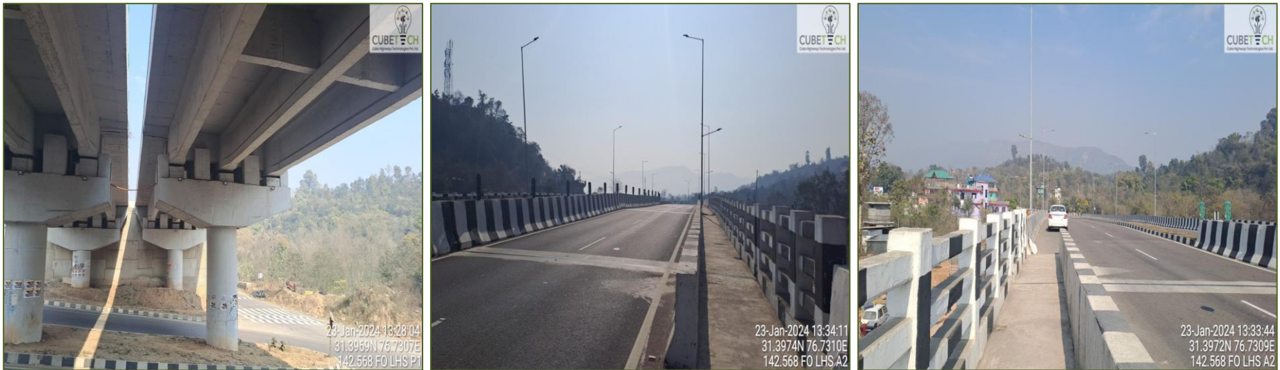
Figure 4-4: Condition of Flyover
