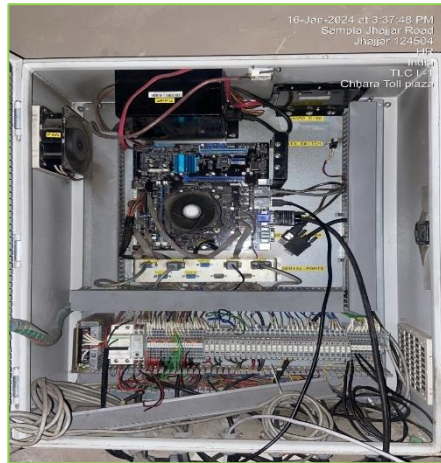
Figure 3-10: Toll Lane Controller at Tunnel
