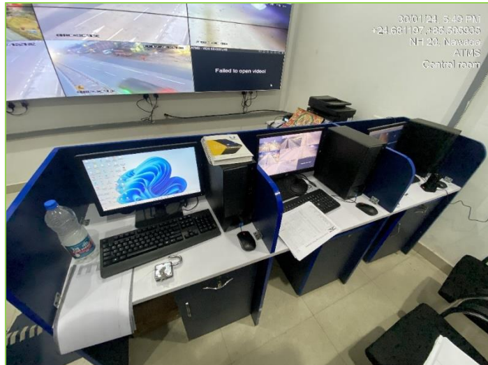
Figure 3-41: Workstations in ATMS control room.
