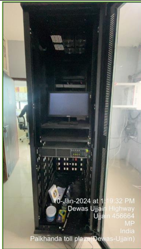
Figure 3-25: Server with rack.
