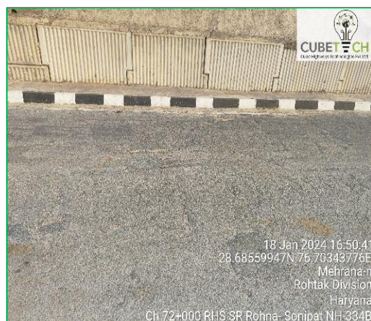
Figure: Alligator Cracks
