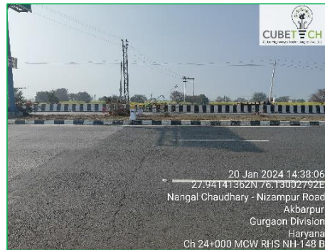
Figure: Tranverse Cracks
