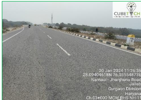
Figure: Longitudinal Cracks
