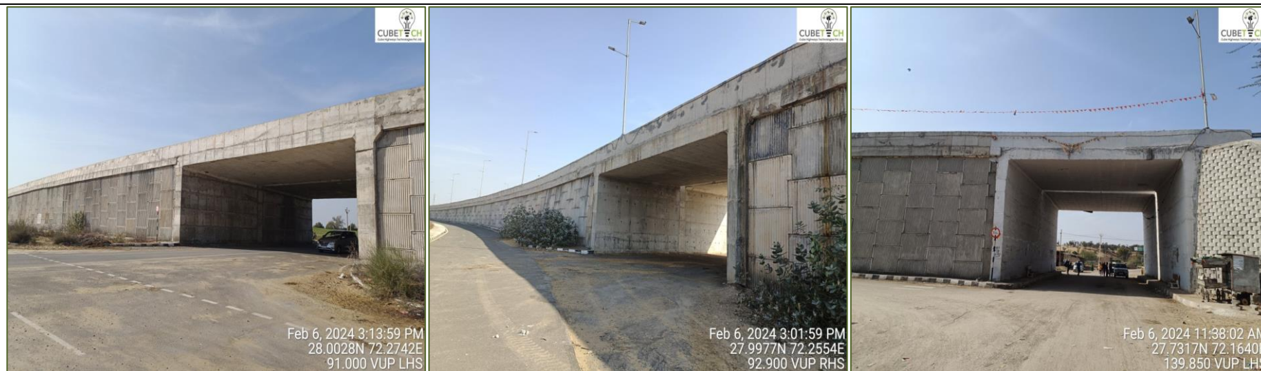
Figure 4-2: Condition of VUPs
