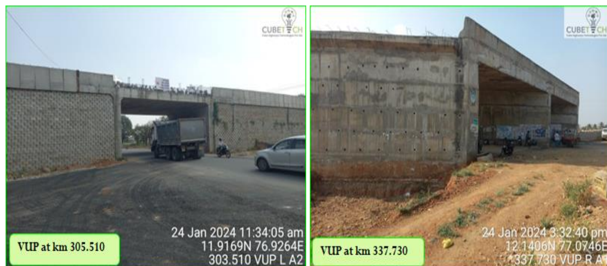
Figure 4-4: Condition of VUPs
