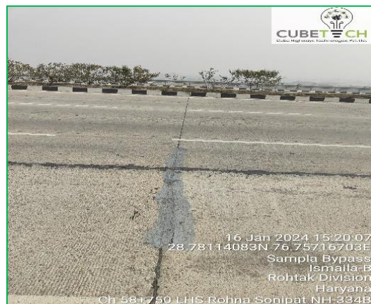
Figure: Spalling of joints
