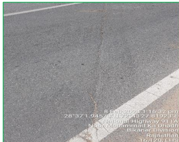
Figure: Transverse cracks
