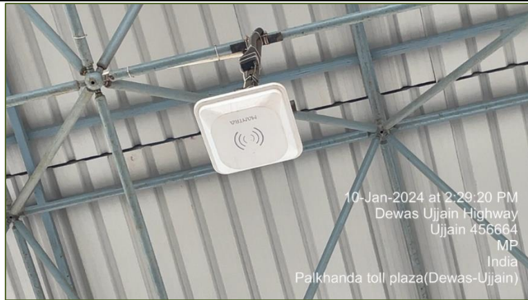
Figure 3-14: RFID ETC Transceiver installed on pole
