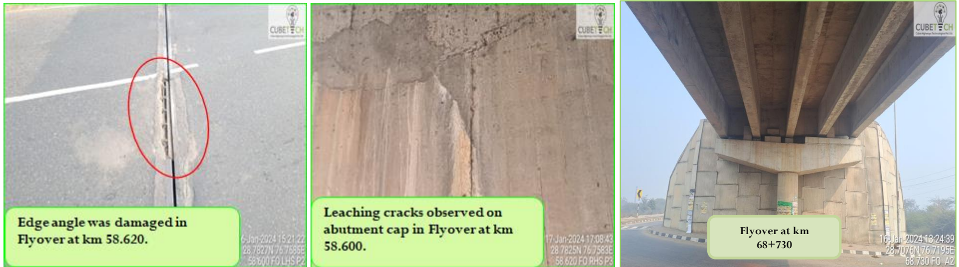
Figure 4-3: Condition of Flyover
