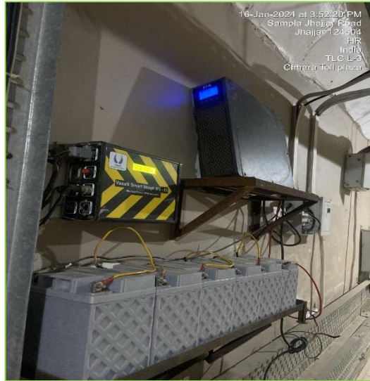
Figure 3-23: Lane UPS in Tunnel.
