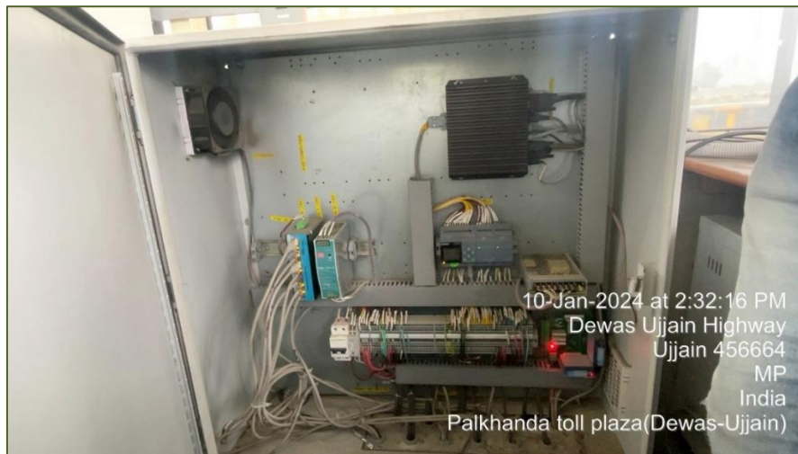
Figure 3-15: Lane Controller at Toll Booth
