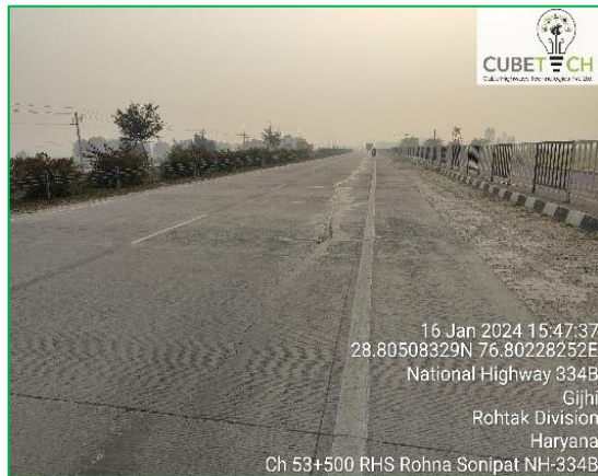
Figure: Longitudinal Cracks
