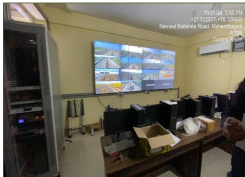
Figure 3-29: Workstations in ATMS control room.
