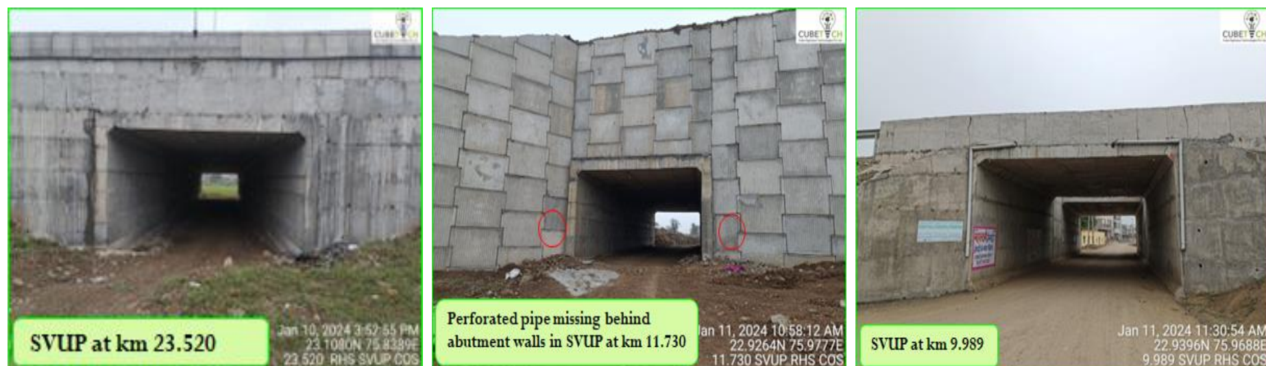
Figure 4-7: Condition of LVUPs
