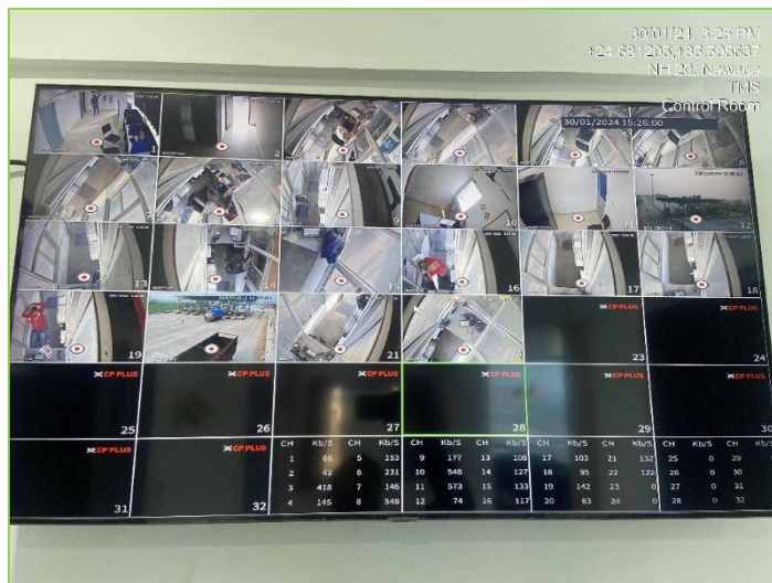
Figure 3-26: CCTV screen at the Toll Plaza Control Room.
