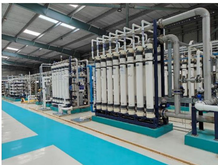
Ultra-pure water generation plant at Unit II
