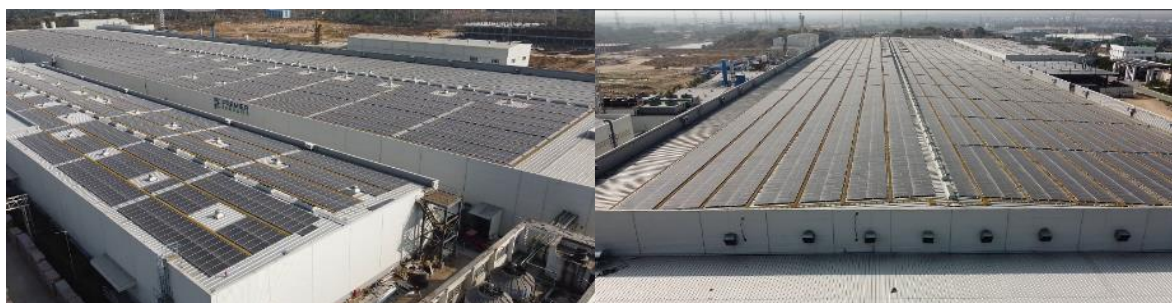
6.61 MW solar rooftop plant
