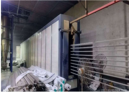
Heat chamber UNIT 1
