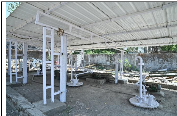
Underground storage tanks
